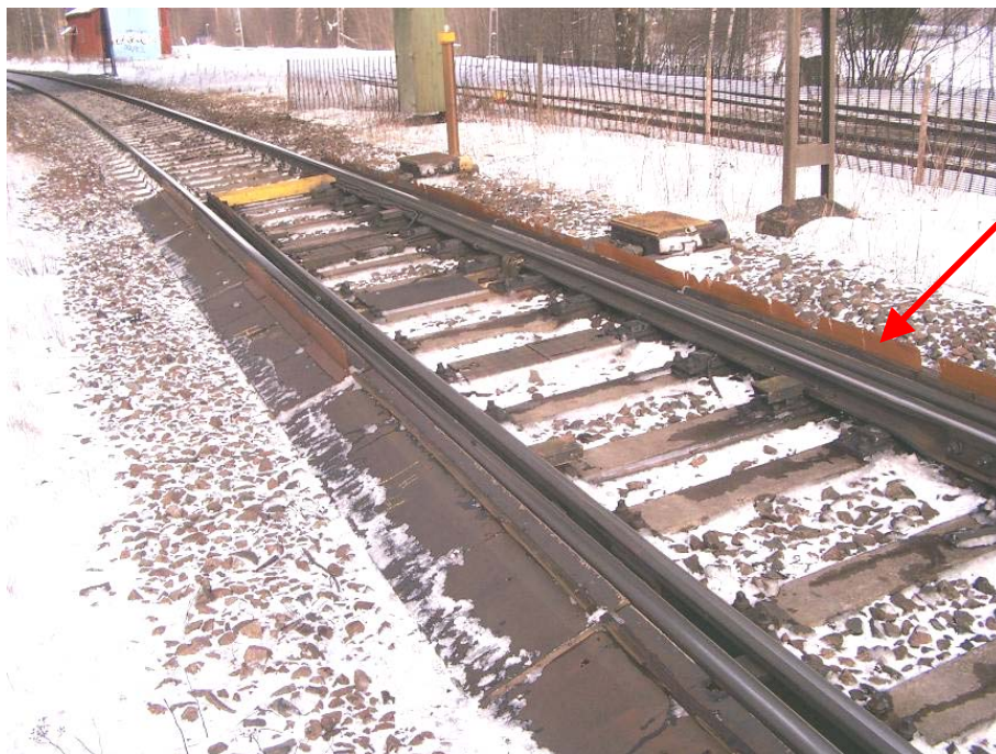
Figure 31. Skutskär. The rubber spoiler as well as the cover outside the rails is shown, see also figure 31. Notice that there are double motors for altering the switch.
