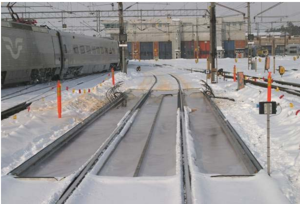
Figure 24. The de-icing facility in Hagalund, Sweden.
