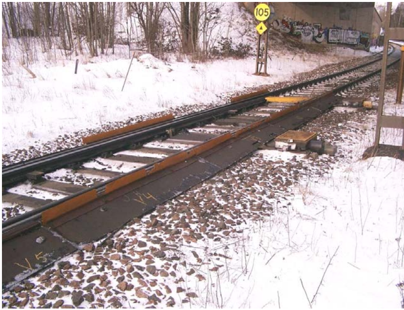
Figure 33. A switch with rubber spoiler and covers outside the main rails. The contacts for positioning control of the tongue can be seen next to the far tongue.
